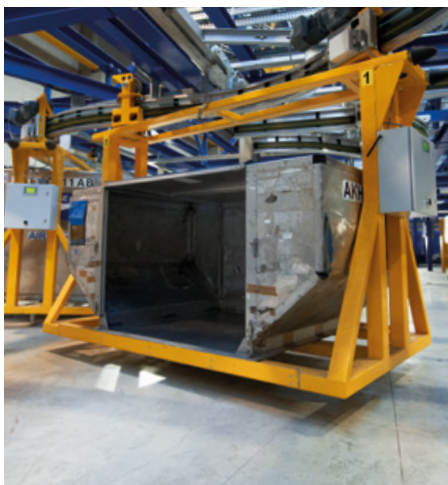
Containers are moved with no operator intervention
