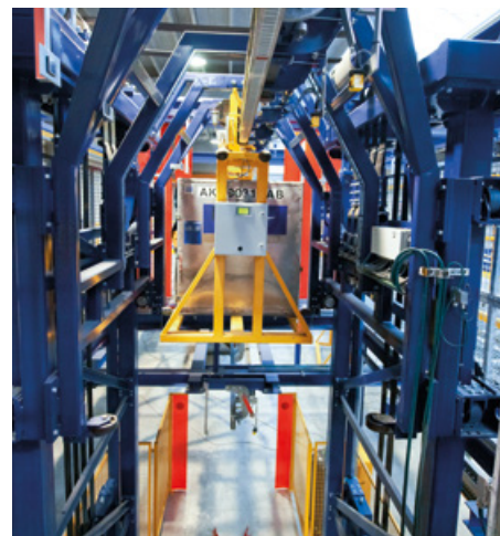
A lift allows ULDs to be moved between destinations on different building levels
